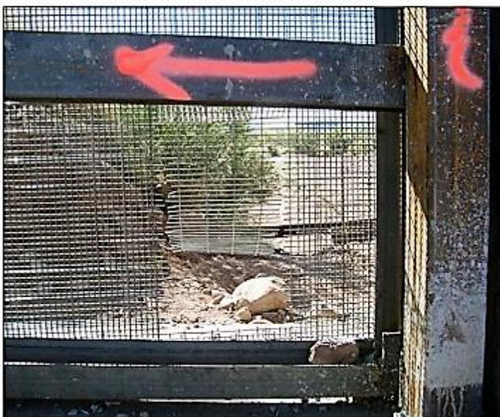
Breach in modern mesh pedestrian fencing
