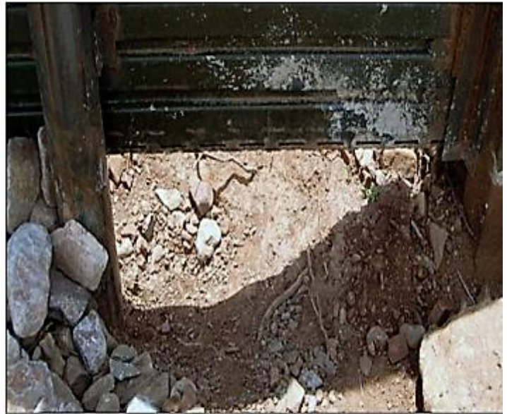
Burrowing activity beneath legacy landing mat pedestrian fence
