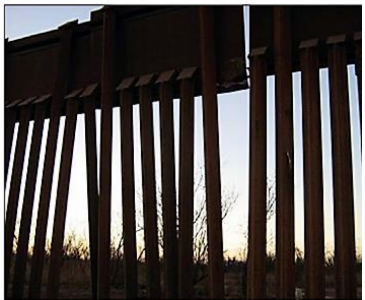
Breach in modern bollard pedestrian fencing
